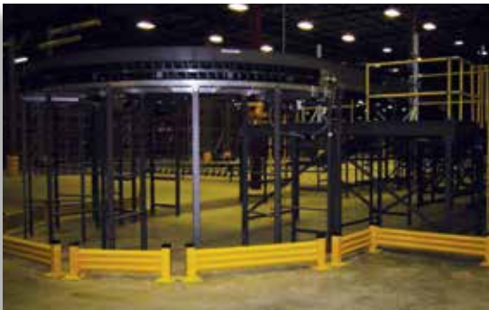
Guarding overhead conveyor
