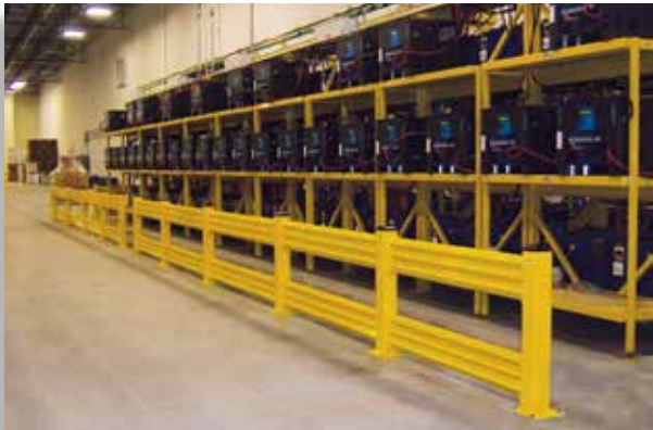
Guarding battery racks
