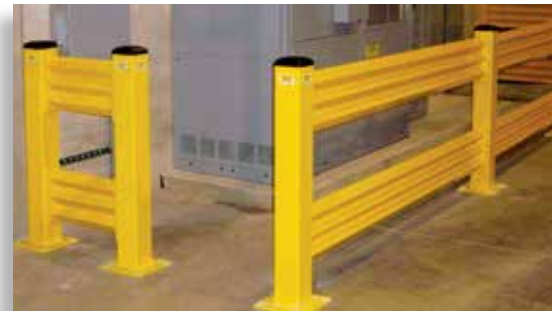
Guarding electrical panels
